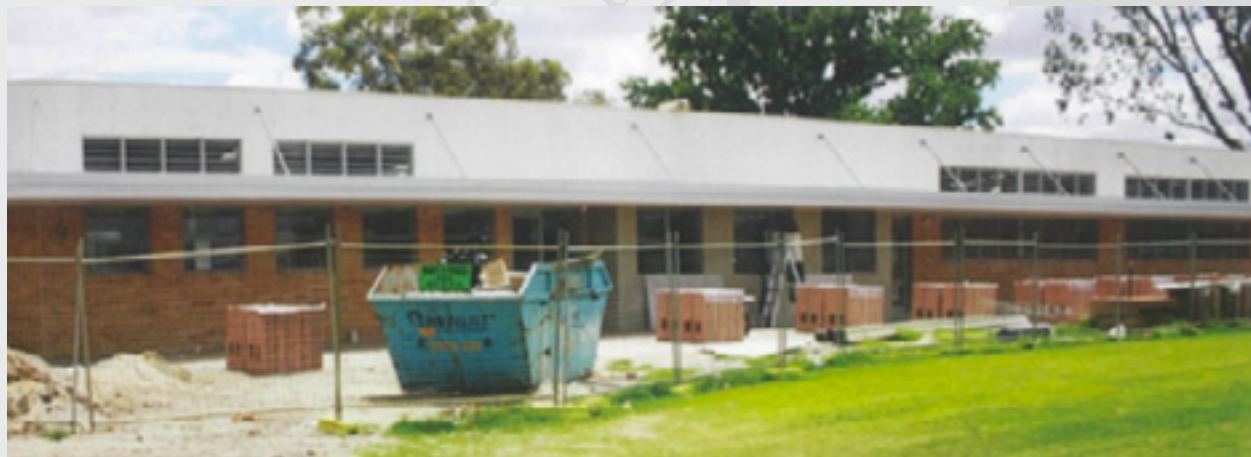
The Floreffe Trade Training Centre and the Cappenburg Language Centre were completed in 2010.
