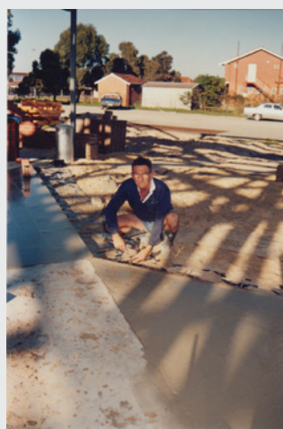
Builder Ben Bianchini hard at work during the construction of the church.
