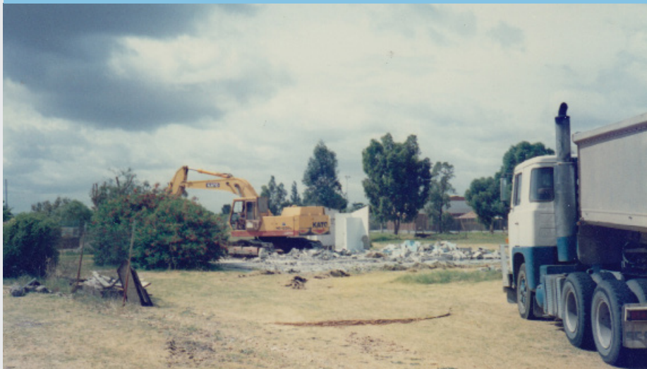
Jeff and Maria Tillemans' house is demolished in preparation for the construction of St Joseph's Priory Church in 1990.
